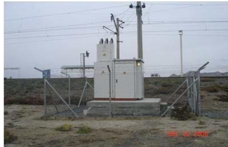
Installation of Sub-stations for: a. SSPS on NREP in Siyazan, Gusar, Sumgait, ST b. SSPS on WREP on PS 2, PS 5 and PS 8
